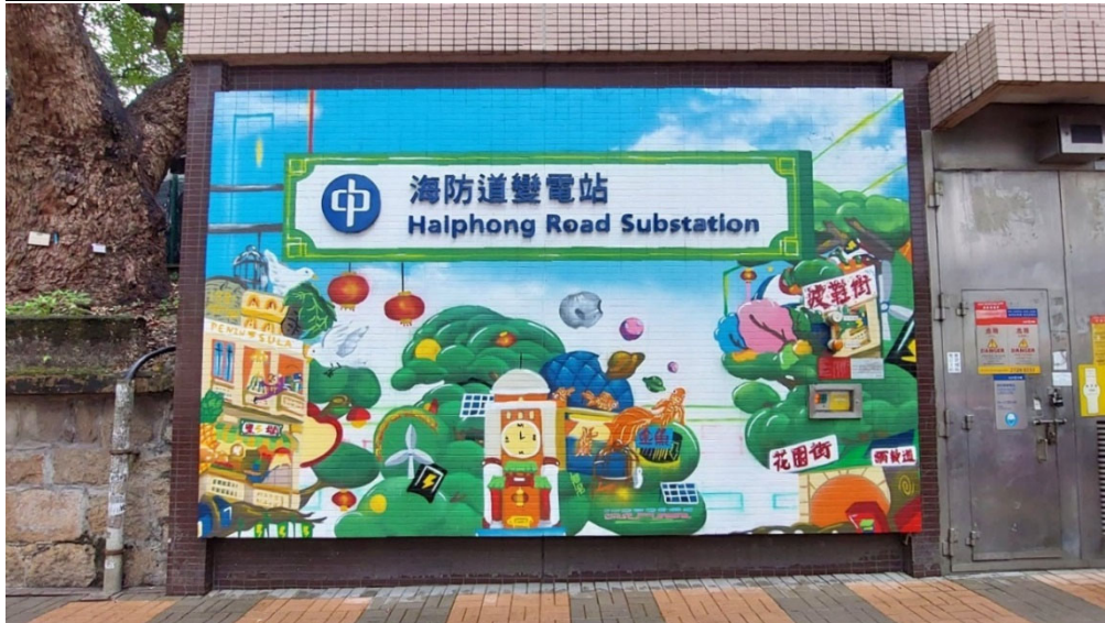
The Haiphong Road Substation in Tsim Sha Tsui is the pilot substation beautified under the CLP Power's Substation Beautification Project last August to promote local culture, history, environmental protection and energy conservation to the public.
