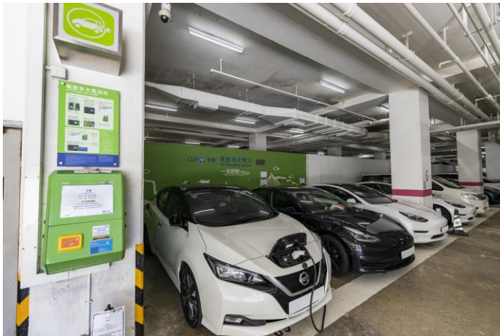
With technical support from CLP Power, Link will provide 3,000 electric vehicle chargers in its car parks by the end of 2024. This collaborative effort will promote low-carbon transport.
