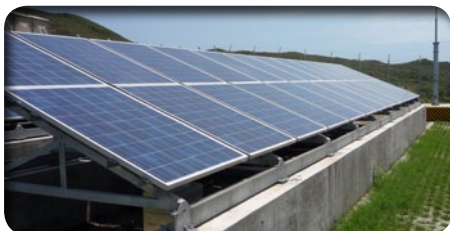
Hong Kong's first commercial-scale standalone renewable energy (RE) system on Town Island
