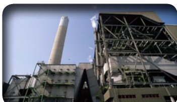
Electrostatic Precipitators at Castle Peak Power Station
